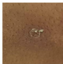
f) partially removed scab
